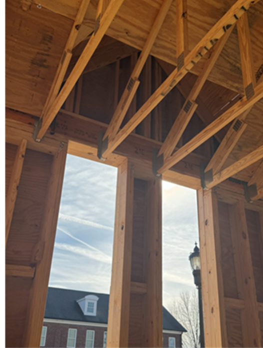
Fitness Room – Joist hanger at window. Spandrel glass scheduled at this elevation.
