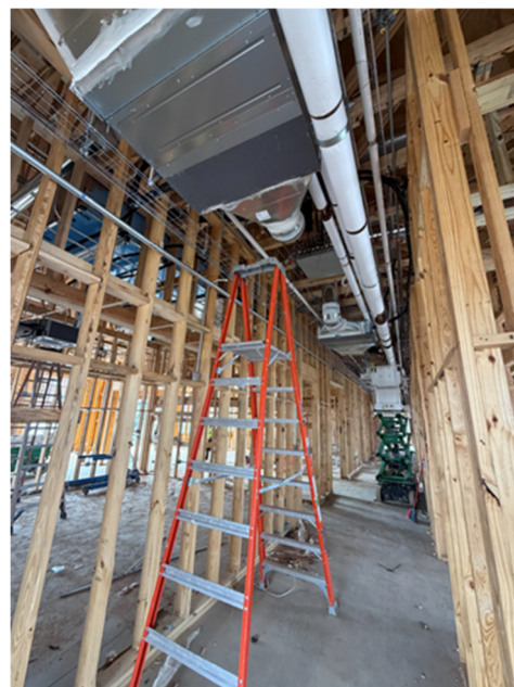
Corridor: Terminal Unit TU-9B installed.
