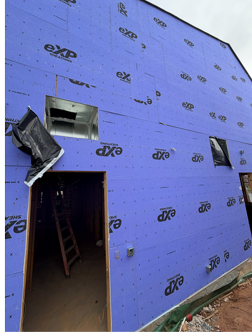
L2: Ensure exterior louver openings are covered and protected.
