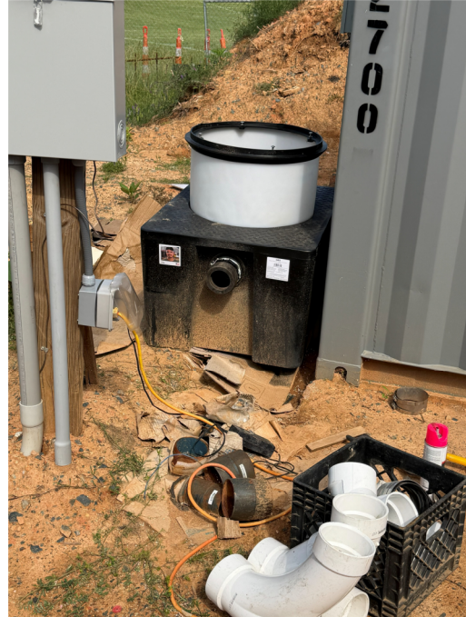
Grease-trap to be installed
