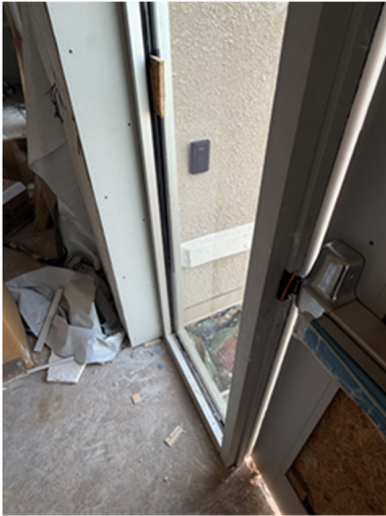
Multi-Purpose storefront side-lite waiting on replacement glass.
